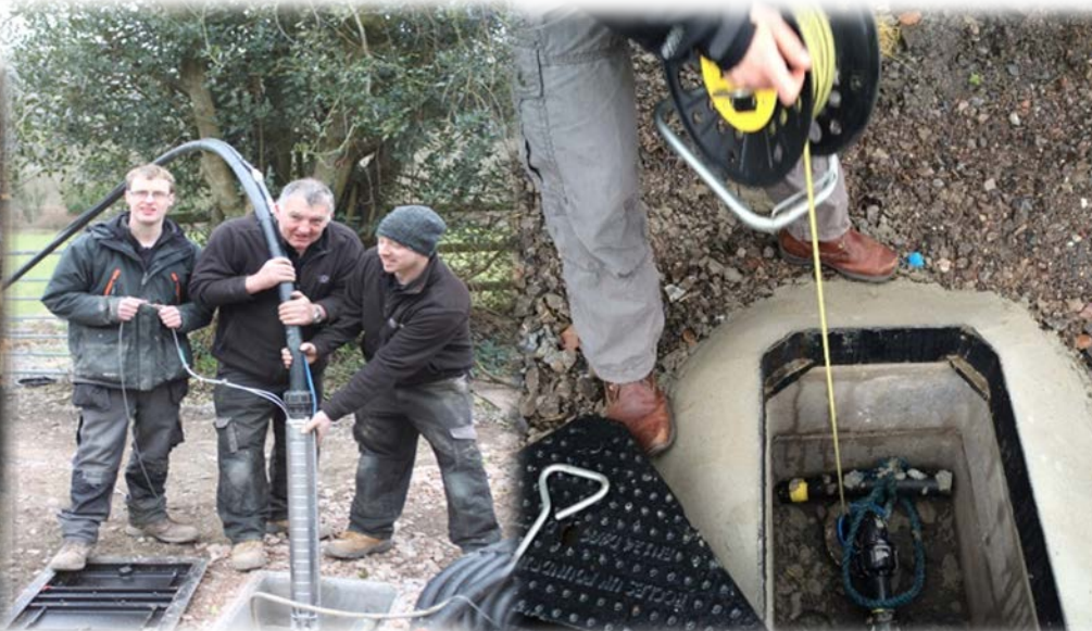
Abstraction and Discharge borehole
