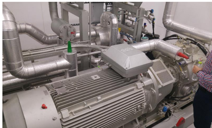
Figure 2: A Heat pump at a district heating plant in Denmark (source: C. Doczekal)
