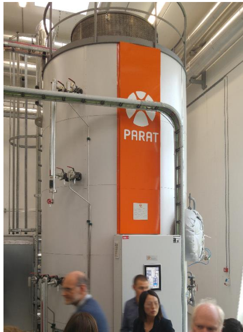
Figure 1: Electrode boiler (10 MW) at a district heating plant in Denmark (source: C. Doczekal)
